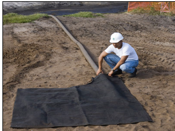
Gravity Bag Filter (Source: http://www.spillcontainment.com )
