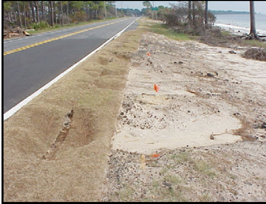
Evidence on sheet erosion and undercutting of sod, August 2005
