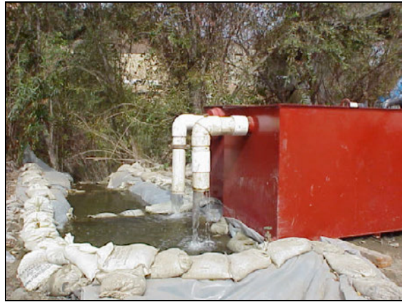
Dewatering Tank (Source: http://www.dot.ca.gov )
