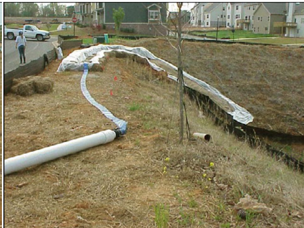
Figure AIII-3: The water was pumped through the pipe mixers and down a jute lined ditch.
