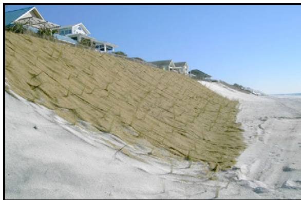
Armoring on beach with jute netting and salt-tolerant vegetation (Source: Foundation Technologies, 2006)
