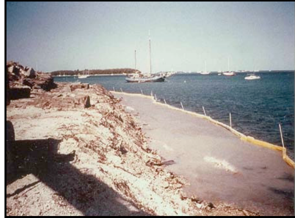
Turbidity barrier and substantial trapped sediment along Maryland coast (Source: IECA, 2006)
