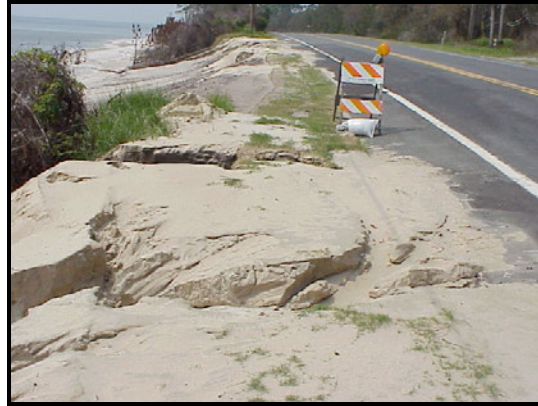
Sheet and gully erosion along shoulder, August 2005
